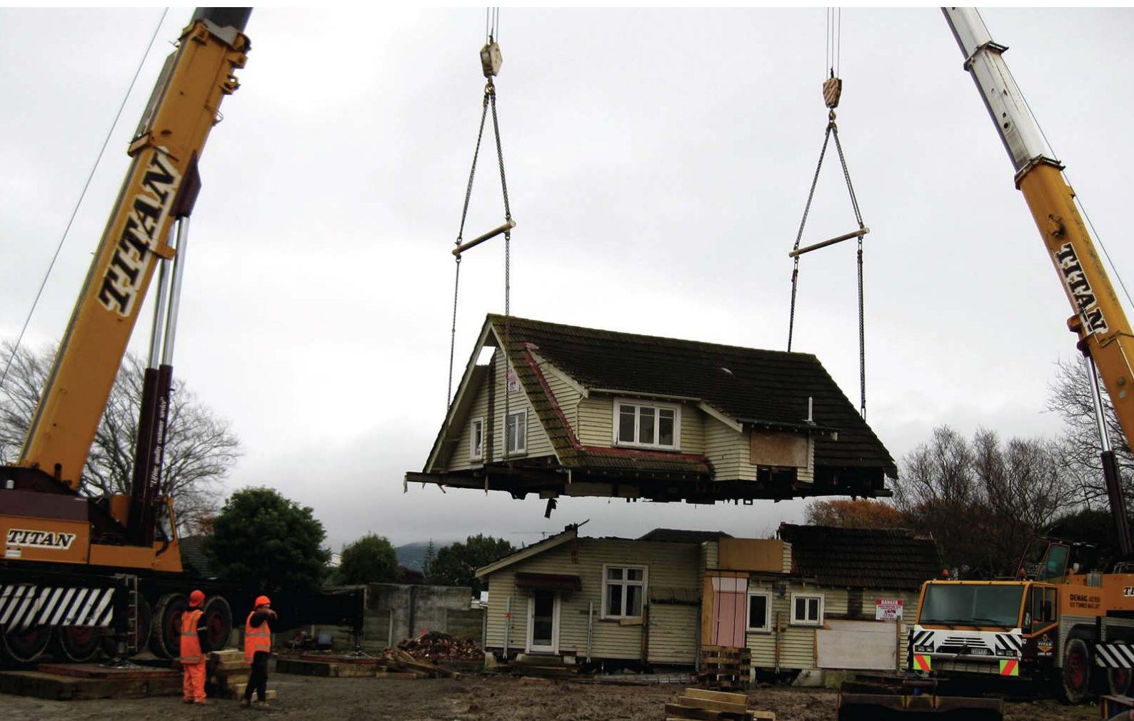
Raising the roof. Titan Cranes' Demag AC615 and Demag AC100 lifting a house at Hutt Hospital, Lower Hutt. (Photo credit: Steven Thomlinson)
