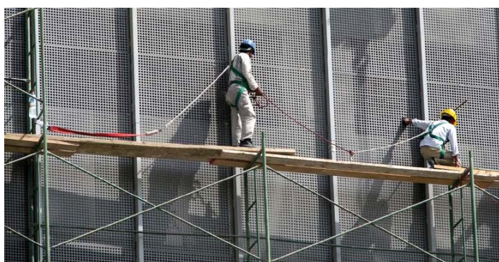
Engineers tried to follow international safety practice but failed as evidenced by the workers wearing harnesses, but doing so dangerously.
