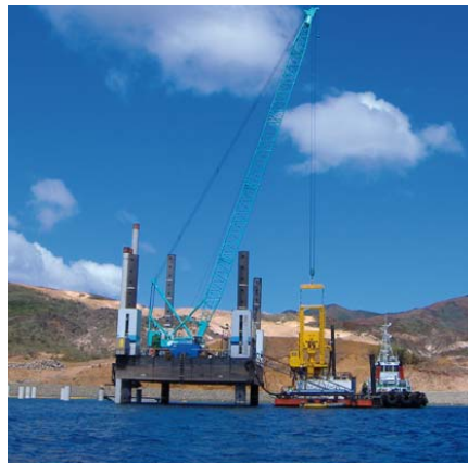
Daniel Smith Industries 250 ton crawler crane on jack-up barge, Goro Nickel Mine, New Caledonia.
